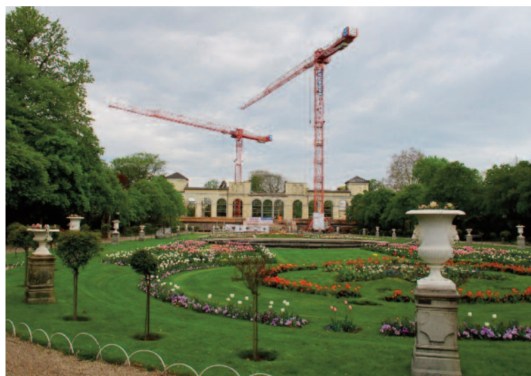
The historic building at the heart of the symmetrically designed botanic garden complex in the Flora – the Botanic Garden of Köln, Germany – reopened in 2014 after a three-year renovation period. Continued communication with all involved stakeholders ensured that the budget for the renovation was secured. (Image: Annette Patzelt)
